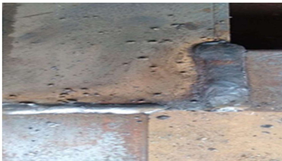
Figure 2. Defect due to Welding Failure
