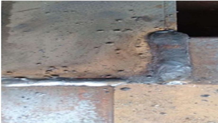
Figure 2. Defect due to Welding Failure
