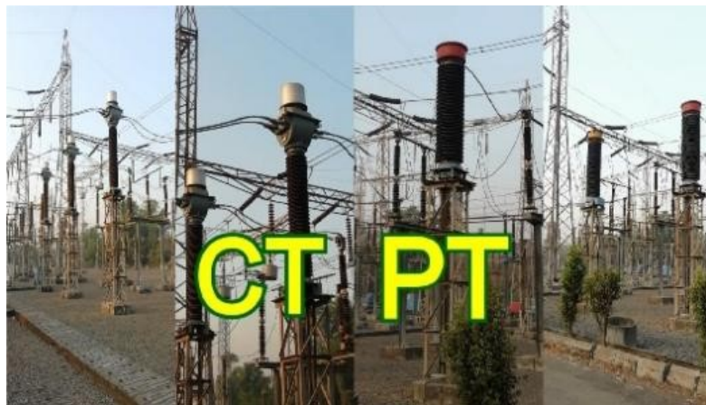
Figure 3. Voltage and Current Sensors
