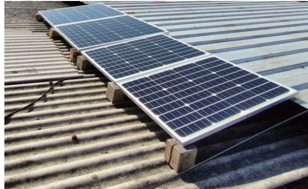
Figure 12. Solar Panel Testing
