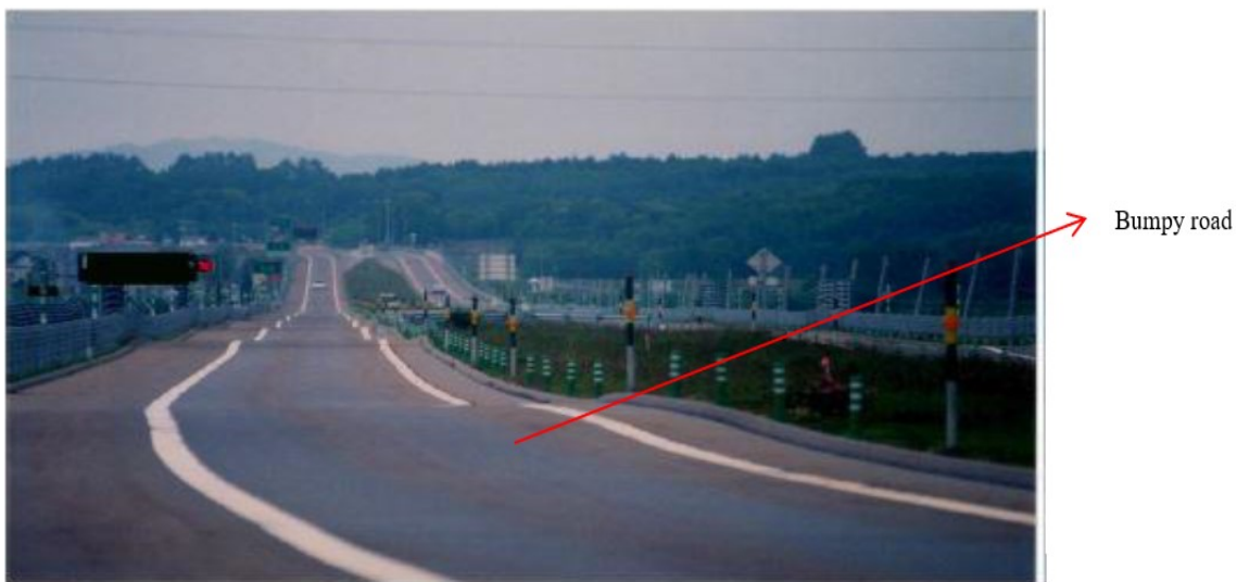
Figure 1. The road settlement failure due to the construction on peaty soil [22]
