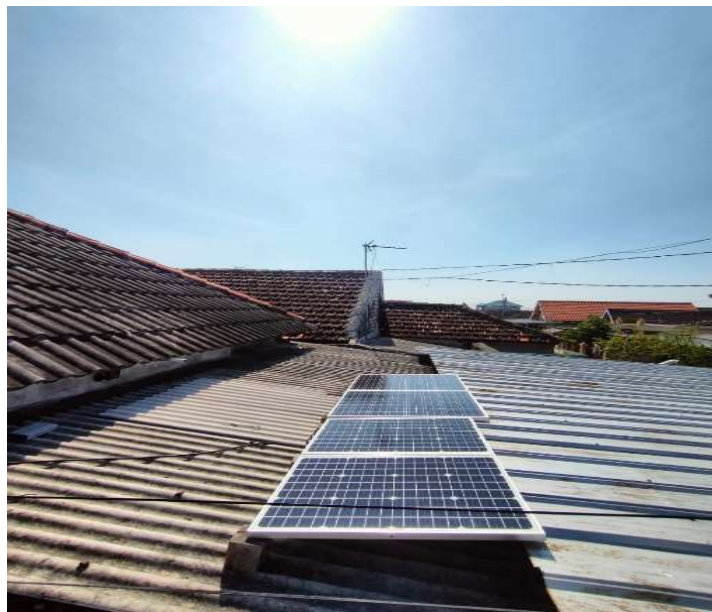
Figure 9. Solar Panel Testing
