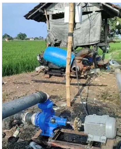
Figure 10. Pump and Motor Placement
